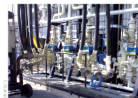
Calibration of a road tanker loading rack in a fuel storage plant
