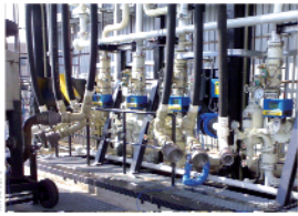
Calibration of a road tanker loading rack in a fuel storage plant
